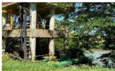
Standerton WTW Vaal River abstraction pump station
