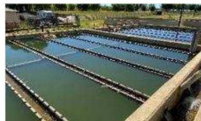
Standerton WTW settling tanks
