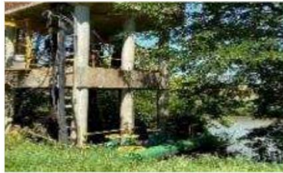
Standerton WTW Vaal River abstraction pump station
